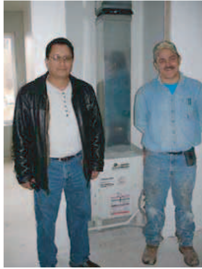
Jorge Lopez of Southwest Minnesota Housing Partnership and Wilcon's Jerome Molitor standing by the heat pump in one of the apartments. These units fit in a small utility closet and provide heating and cooling for the individual apartments. A programmable thermostat in each unit allows tenants to control their own environment.
